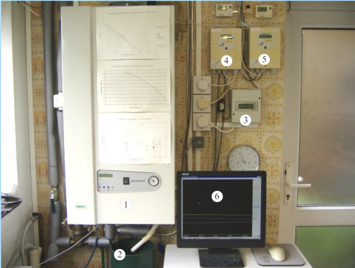
1 Boiler, 2 Rain Gauge, 3 Electricity sub-meter, 4 Heat Meter-Boiler, 5 Heat Meter-DHW, 6 Screen of Data Logger PC.
